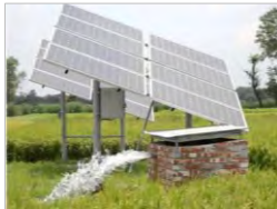
Solar lift irrigation
