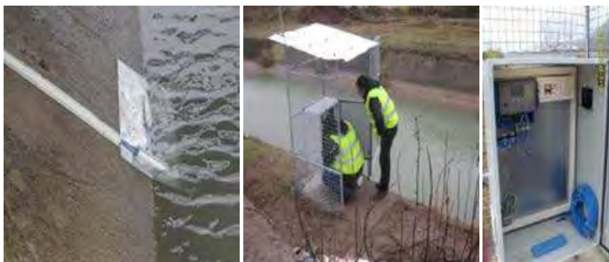
Figure 2. Installation of ultrasonic water measurement in canal irrigate
