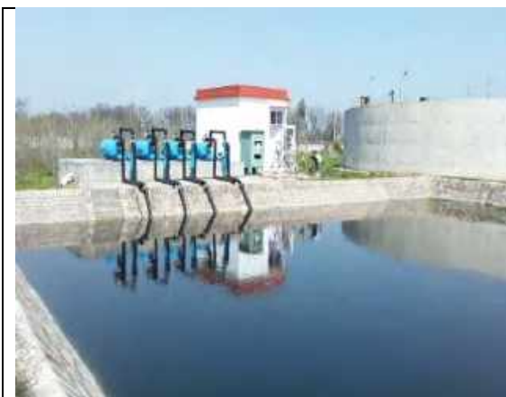
Photo 1. TWW tank, Irrigation Control Head Unit
