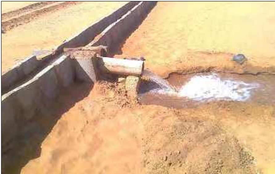
Plate (1): A lined section and field out-let pipe made of local aggregates
