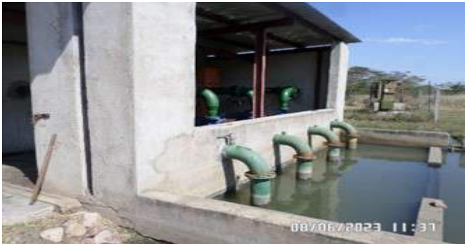
Figure 11: Water Reuse Pump Station
