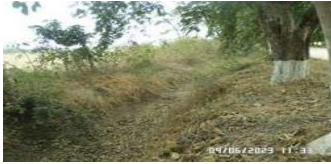
Figure 21: Storm drains at Lusitu Banana Scheme
