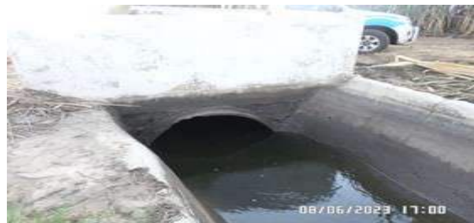
Figure 26: Asbestos Pipe ( Source: Author )
