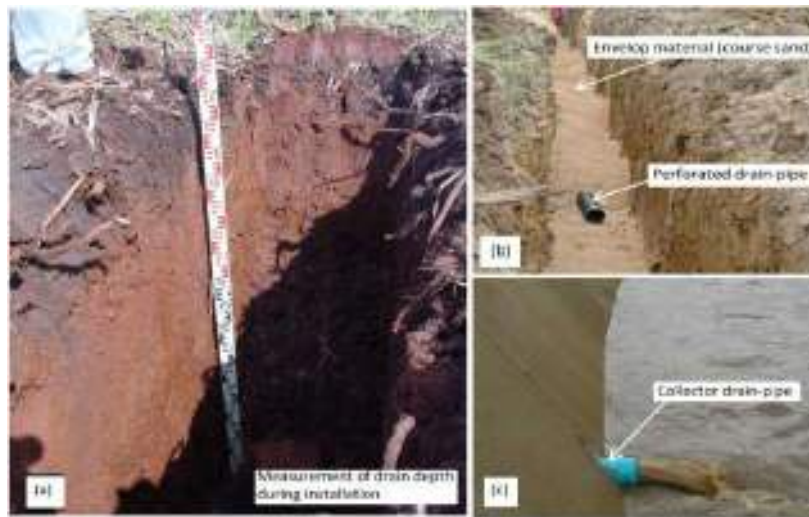
Figure 1. Details of the existing subsurface drainage system ((a) excavation of trenches at the required depth, (b) installation of perforated subsurface drain pipes, and (c) a collector drain pipe discharging into an open drain)
