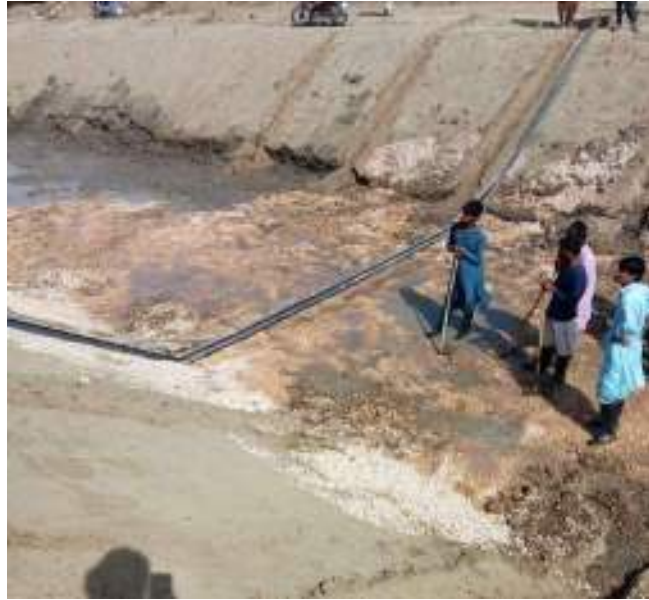
Figure 13: Observed Sloughing during Bed Formation
