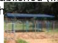
Figure 3: Solar-Powered irrigation system.
