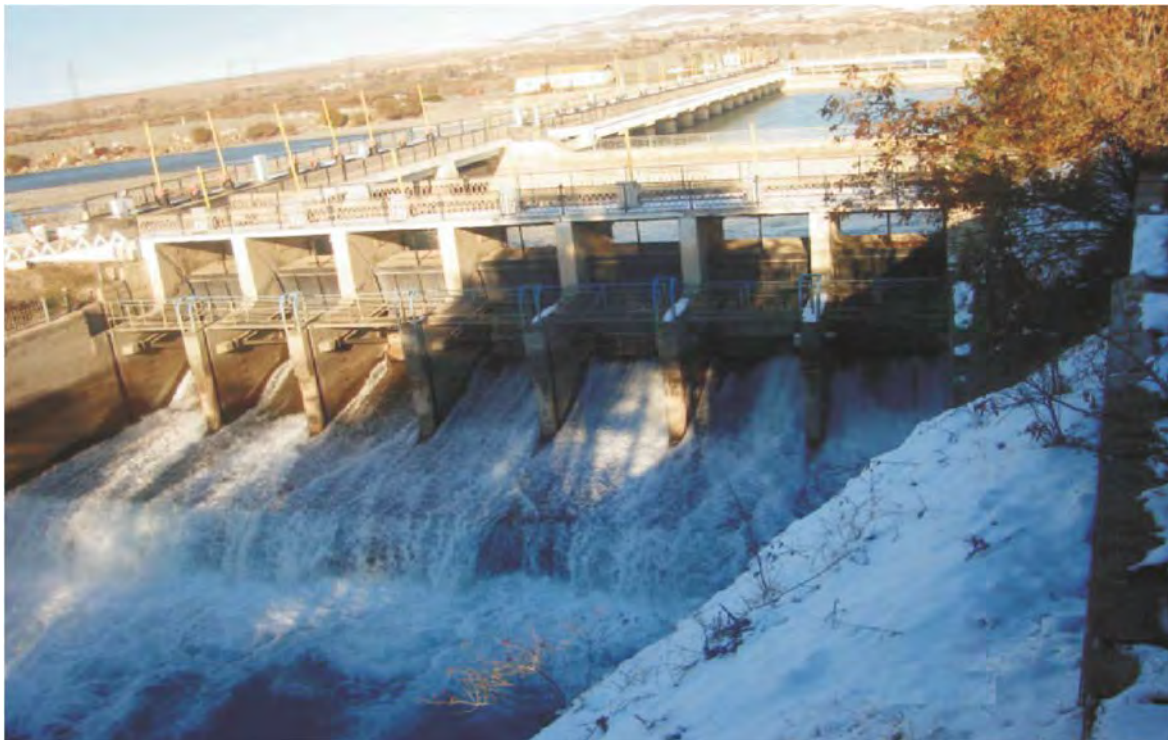
Figure 5. The Ravatkhodja Hydrostructure on the Zarafshan River
