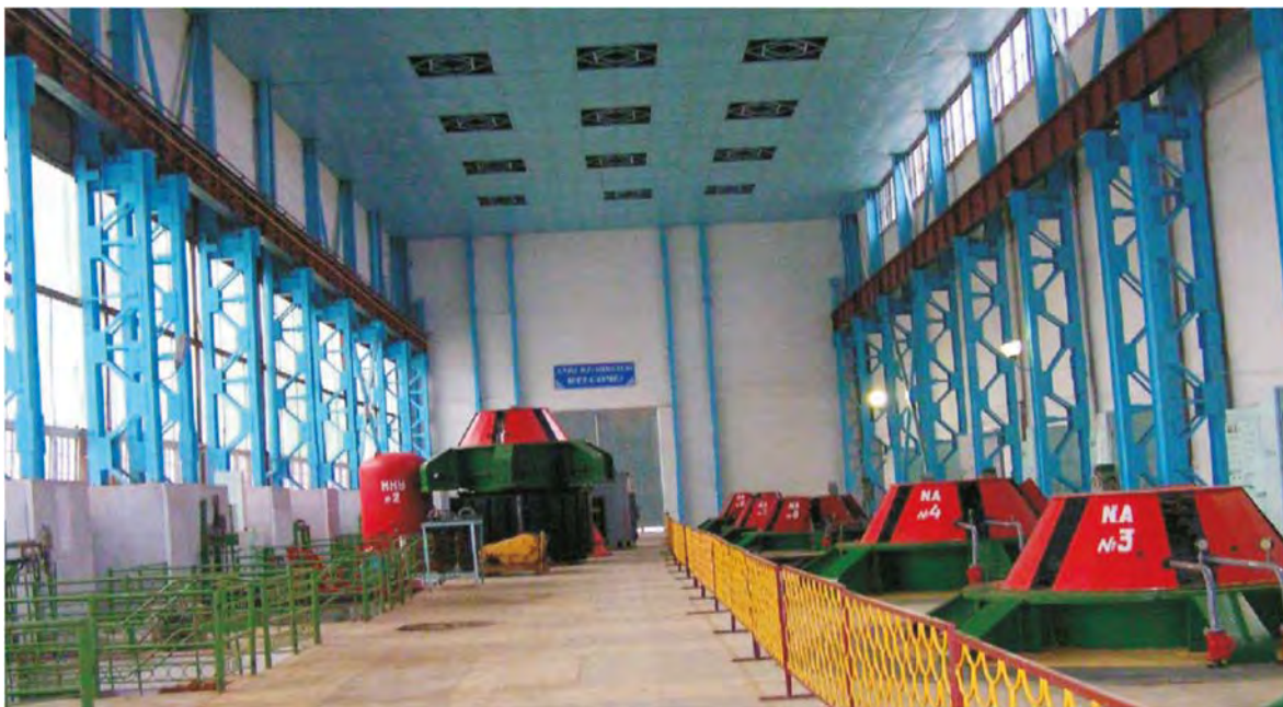
Figure 8. Pumping hall of the Babatag Pumping Station in Surkhadarya province
